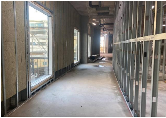
The Baird Family Hospital North Side Internally - External Wall (left) and dry wall partitions on the right on north first floor corridor
