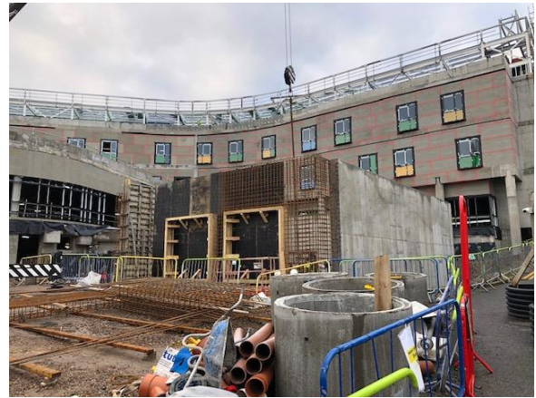
The Baird Family Hospital West Side - Preparation for concreting the generator housing
