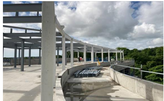
Formation of steelwork to create Engineering Plant Space on top floor of The Baird Family Hospital
